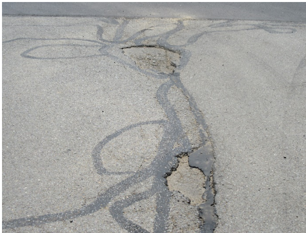
Asphalt pavement deterioration at Moline Place
