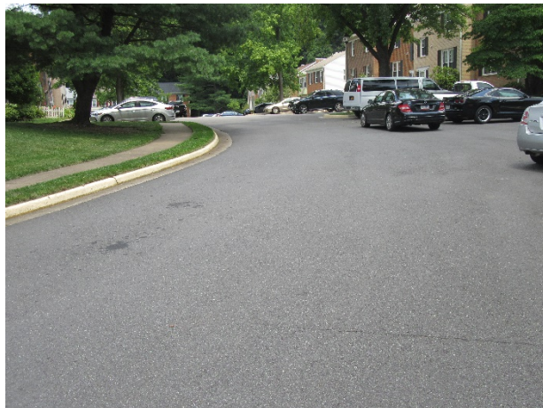
Asphalt pavement at Brandeis Way; we note minor cracks
