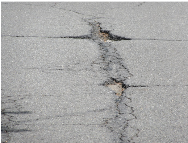
Asphalt pavement deterioration at Euclid Way
