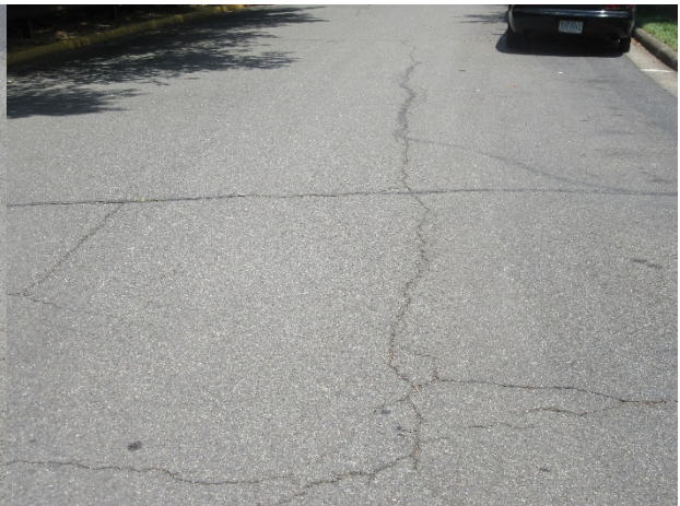
Asphalt pavement cracks at Euclid Way
