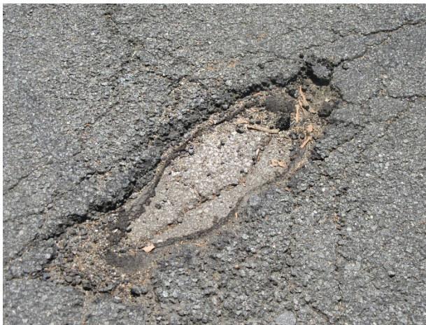
Asphalt pavement deterioration at Dampier Court
