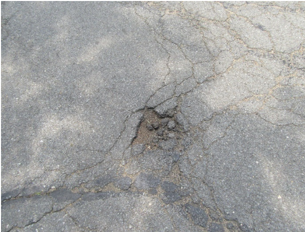
Asphalt pavement deterioration at Luce Court
