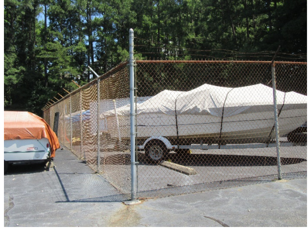
Chain link fence at the pool house parking area; we note rust
