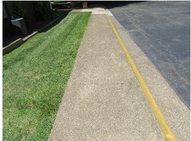
Concrete sidewalk spall
