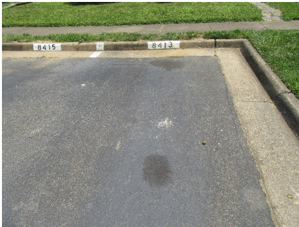
Asphalt pavement vehicular fluid stains at Eucalyptus Way
