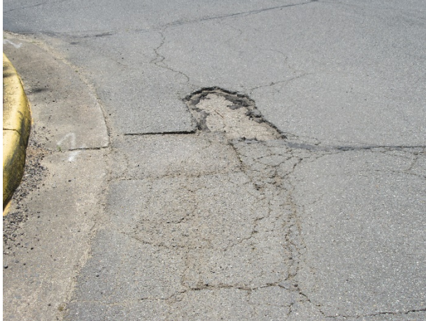
Asphalt pavement deterioration at Red Ash Court
