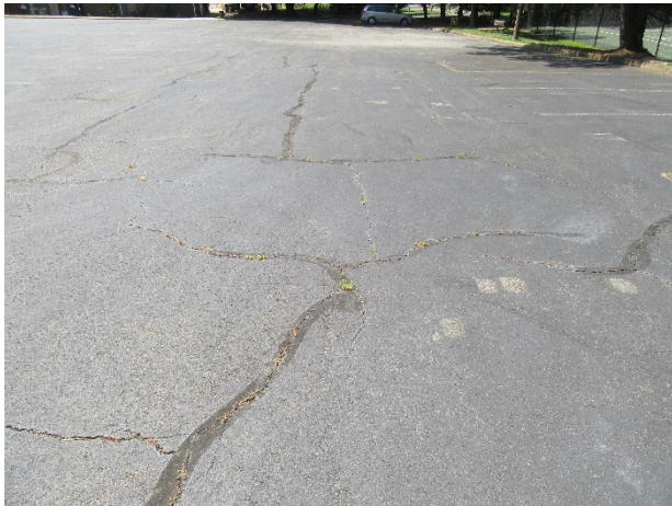
Asphalt pavement cracks and previous repairs
