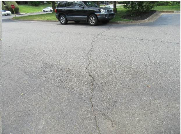
Asphalt pavement cracks at Marconi Court
