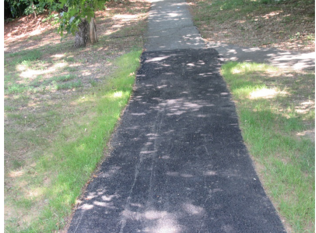
Walking path at Location 1B partial replacement; we note cracks
