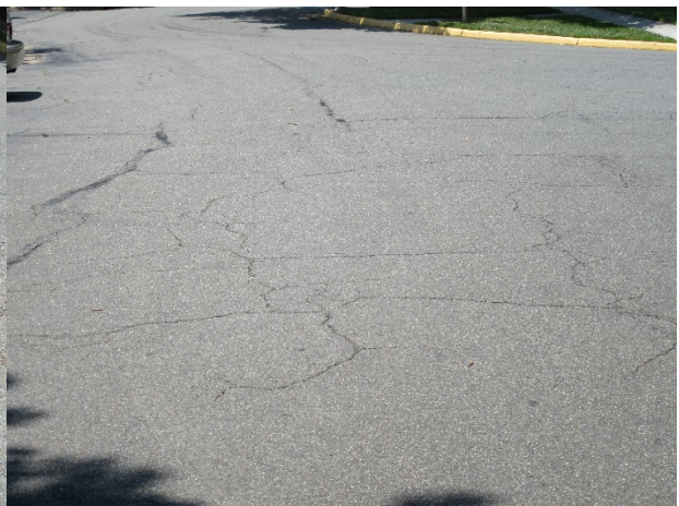
Asphalt pavement cracks at Matisse Way
