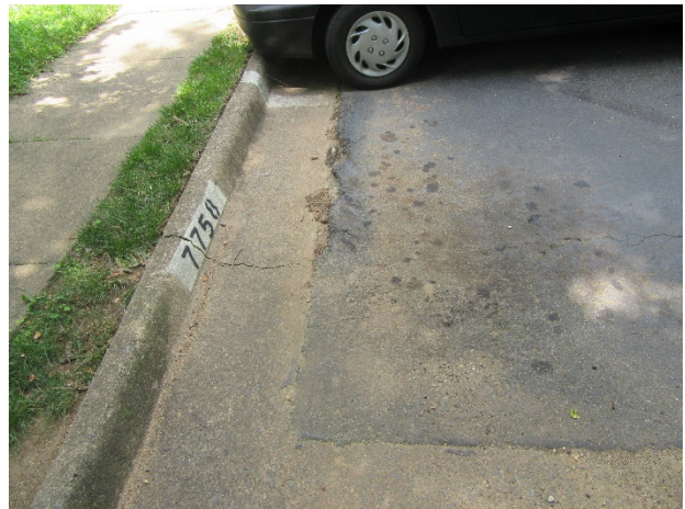
Concrete curb and gutter crack
