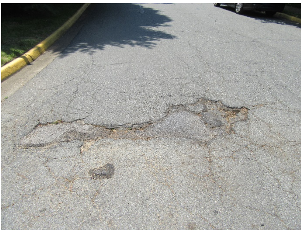
Asphalt pavement deterioration at Rowanta Way
