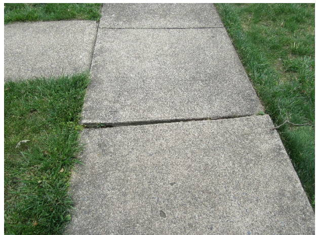
Concrete sidewalk settlement
