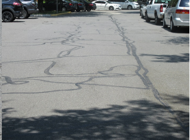
Asphalt pavement previous repairs at Moline Place
