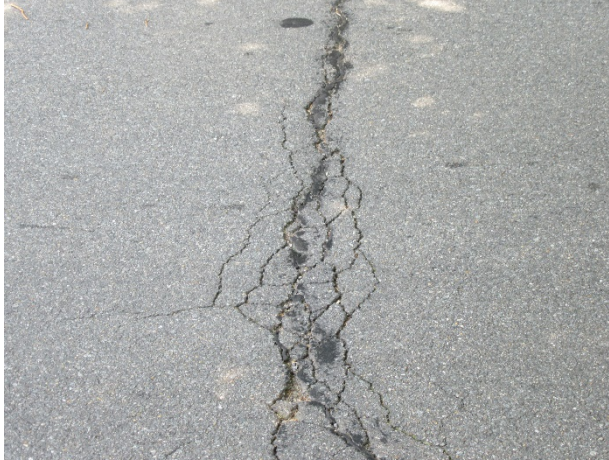
Asphalt pavement deterioration at Matisse Way
