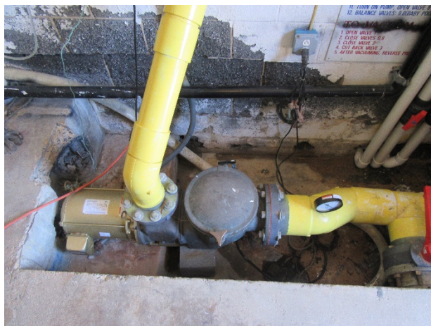
Pool mechanical equipment
