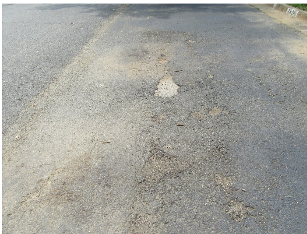
Asphalt pavement deterioration at Marconi Court
