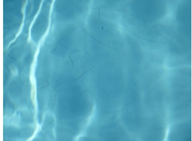
Plaster finish cracks at the main pool
