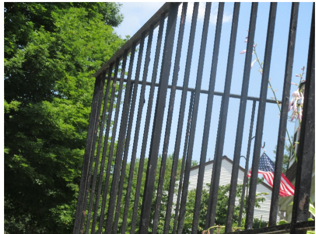
Railings finish deterioration
