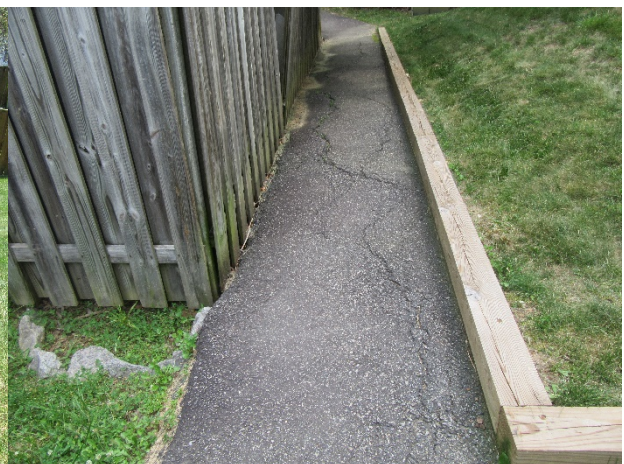
Walking path cracks at Location 2A
