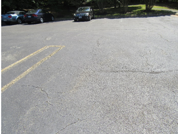
Asphalt pavement parking area; we note cracks and previous repairs
