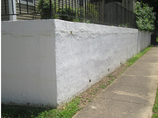
Concrete retaining wall; we note coating cracks
