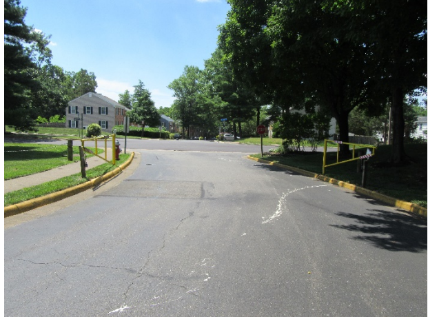
Asphalt pavement access drive; we note patches
