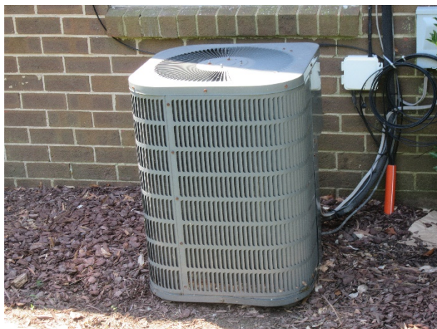
Pool house condensing unit
