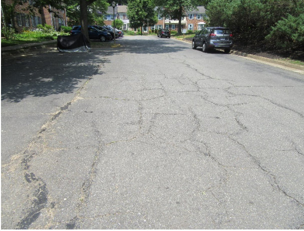
Asphalt pavement cracks at Lemoyne Lane
