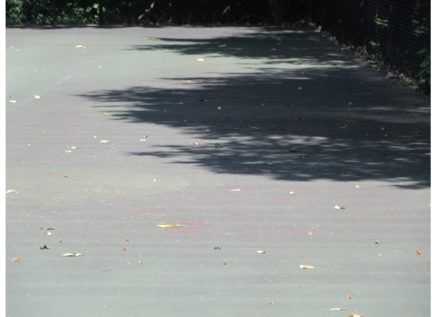
Tennis Courts discoloration
