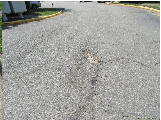
Asphalt pavement cracks at Dampier Court
