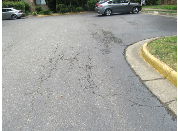
Asphalt pavement cracks and deterioration at Jenner Court
