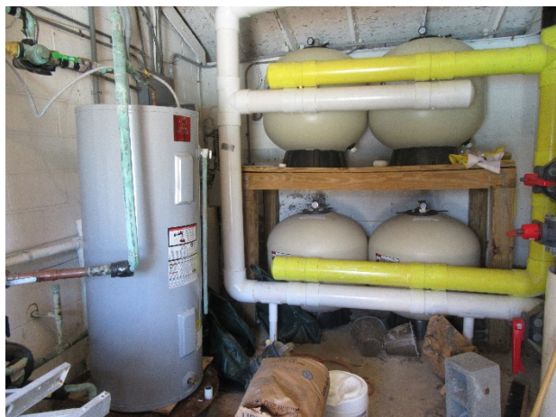
Pool mechanical equipment
