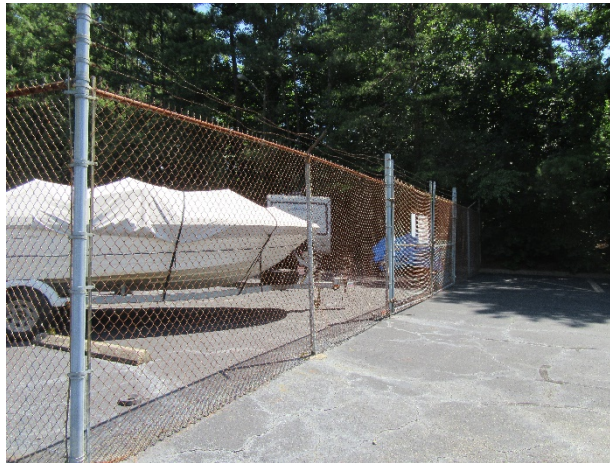
Chain link fence at the pool house parking area rust
