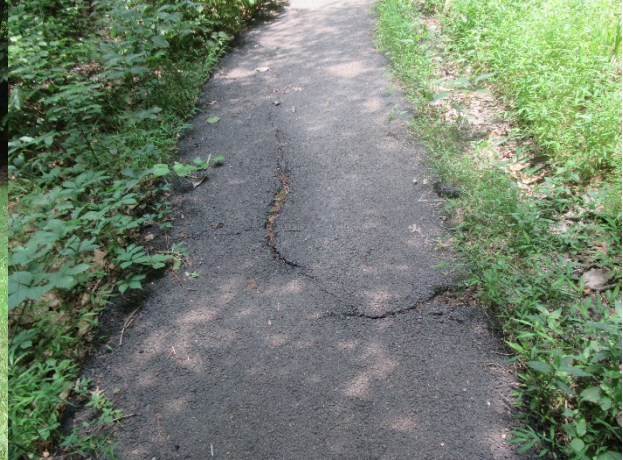
Walking path cracks at Location 2B
