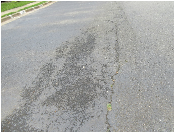
Asphalt pavement cracks and deterioration at Jenner Court
