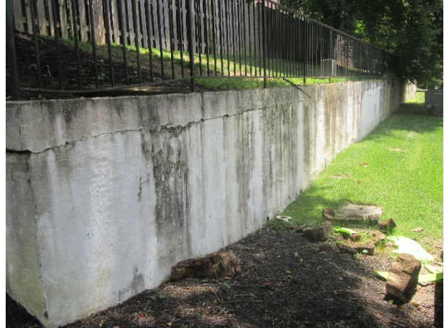
Concrete retaining wall cracks and finish deterioration
