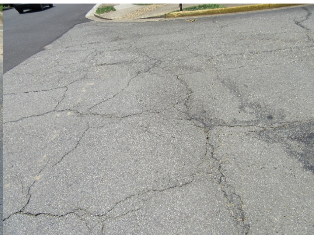
Asphalt pavement cracks at Lemoyne Lane
