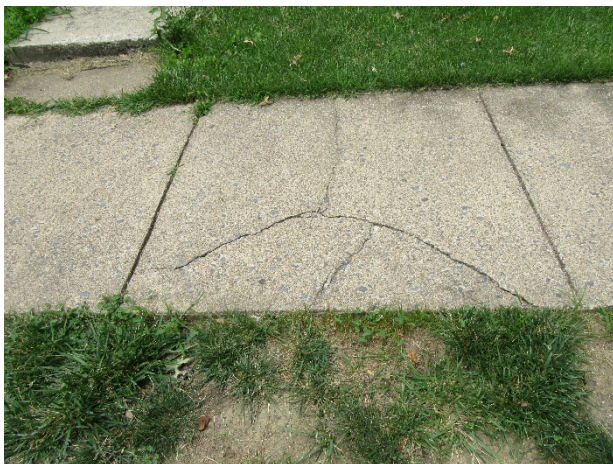
Concrete sidewalk cracks
