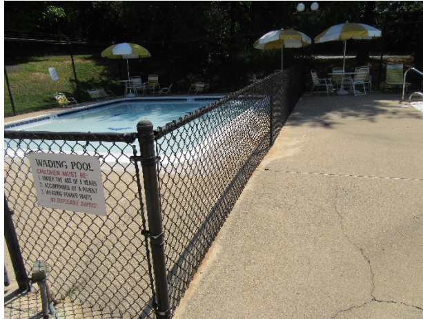
Pool concrete deck cracks
