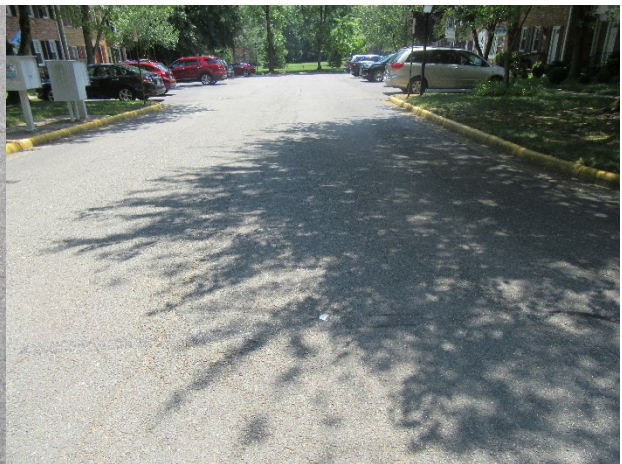
Asphalt pavement at Getty Court; we note minor cracks
