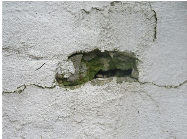
Concrete retaining wall deterioration
