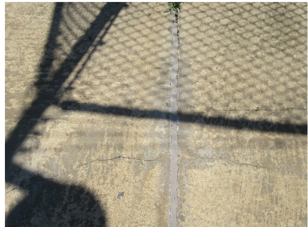
Pool concrete deck previous repairs
