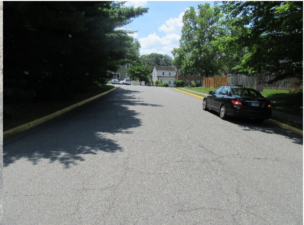
Asphalt pavement cracks at Rowanta Way
