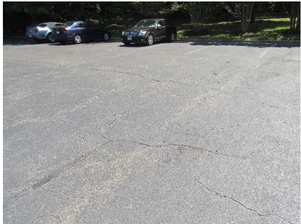
Asphalt pavement cracks and previous repairs
