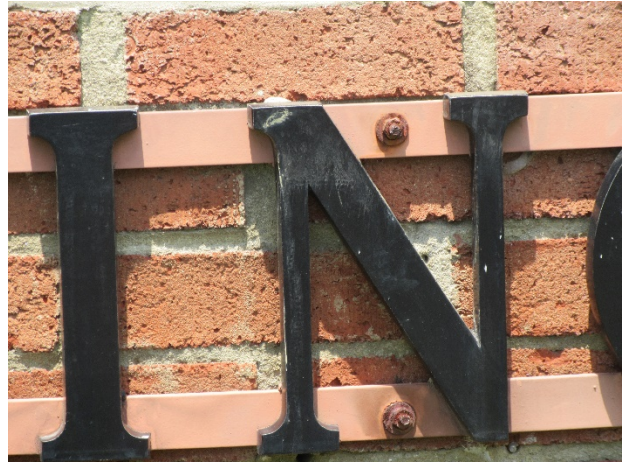
Entrance monument fasteners rust
