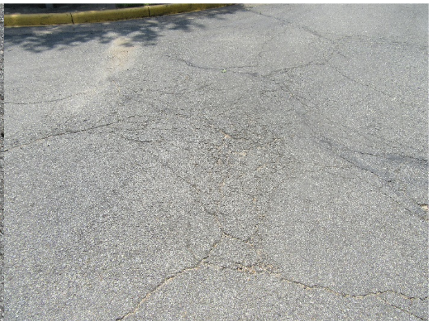
Asphalt pavement cracks at Red Ash Court
