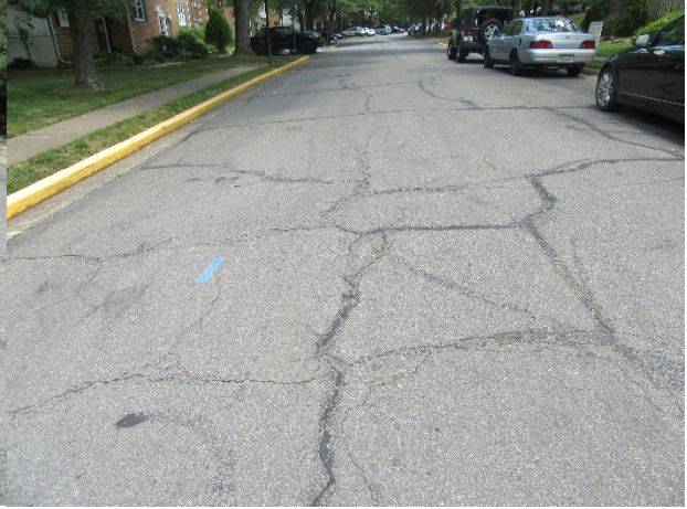
Asphalt pavement cracks at Luce Court; we note previous repairs
