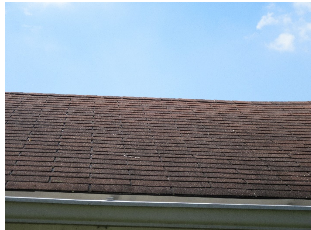
Asphalt shingle roof discoloration
