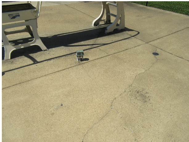
Pool concrete deck cracks
