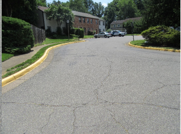
Asphalt pavement cracks at Eucalyptus Court
