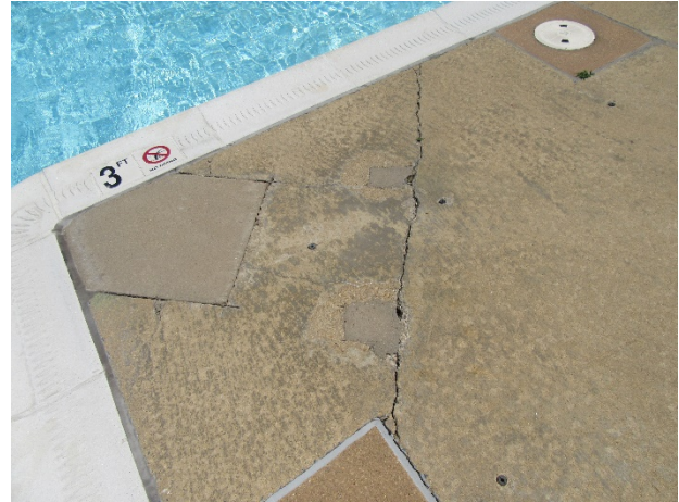
Pool concrete deck crack
