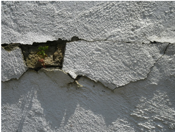
Concrete retaining wall coating deterioration
