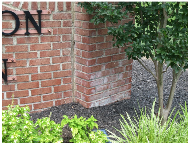
Entrance monument efflorescence
