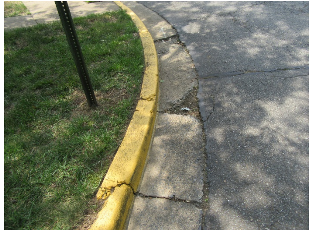
Curb and gutter cracks and deterioration
